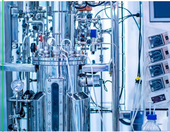
Check Valves are useful in bioreactors to help control the pressure and gas mixing operations.
